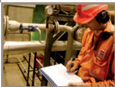
(ABOVE LEFT) Changes are near completion for CSR's ethanol distillery at Sarina, Queensland, to produce fuel ethanol.
