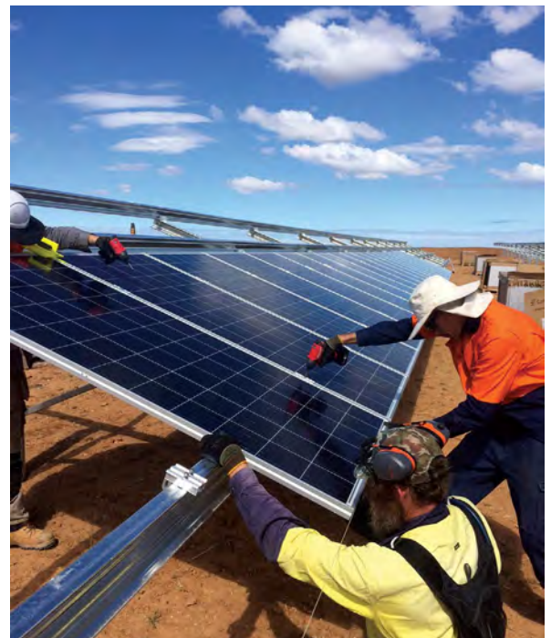
THE SOLAR FARM AT GOLDEN GROVE IN SOUTH AUSTRALIA IS A $2 MILLION INVESTMENT, CONSISTING OF 3,080 SOLAR PANELS AND 31 INVERTERS.
